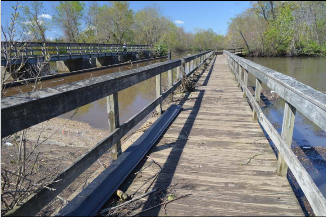
Photograph 1 – Debris from Overtopping at D & R Canal Aqueduct
