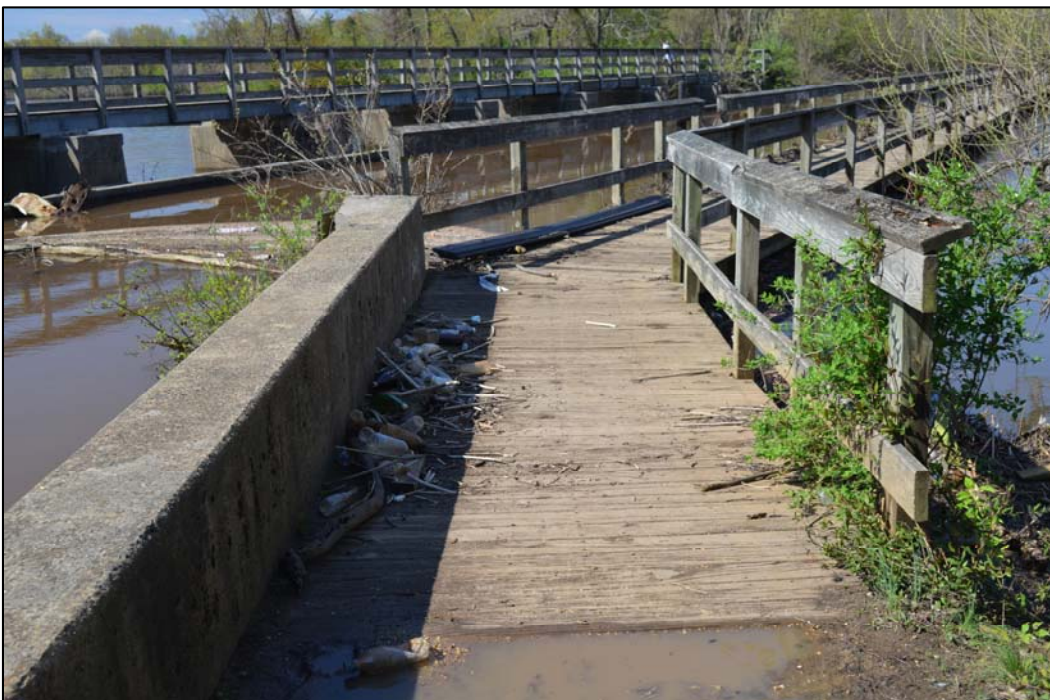
Photograph 2 – Debris from Overtopping at D & R Canal Aqueduct
