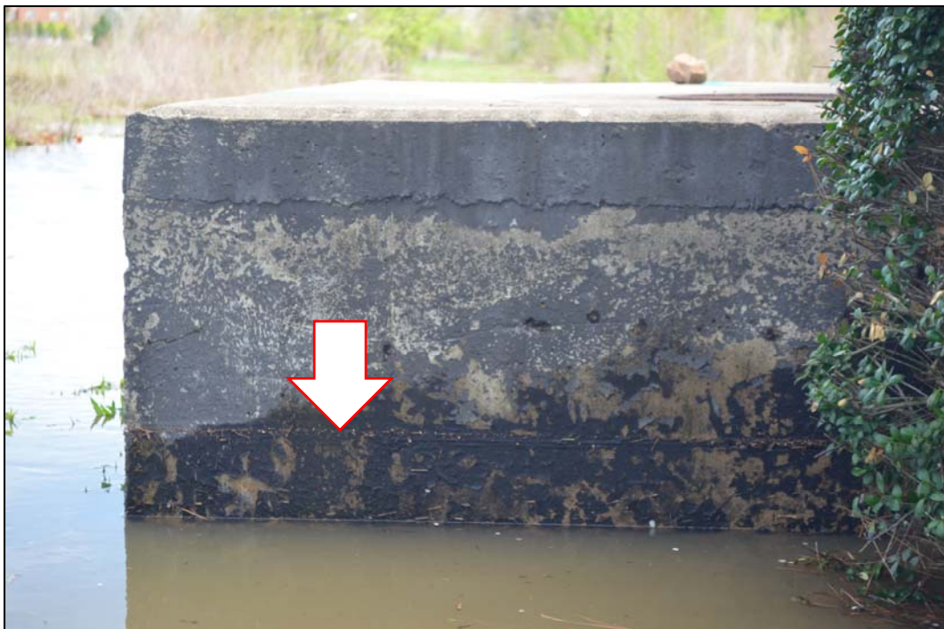
Photograph 6 – High Water Mark Upstream of U.S. Route 1 Bridge
